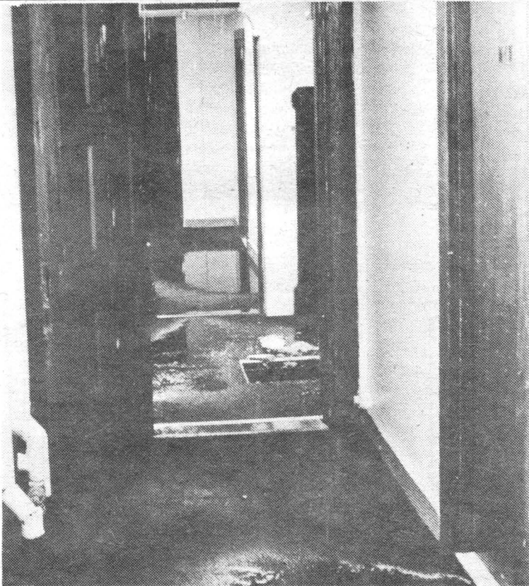
Water from the broken pipe soaks the first floor at Seabury.
