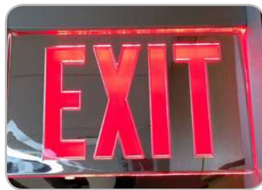
Figure 36: UNO should expect noticeable energy savings by replacing its older exit signs with newer ones that utilize LED technology.
