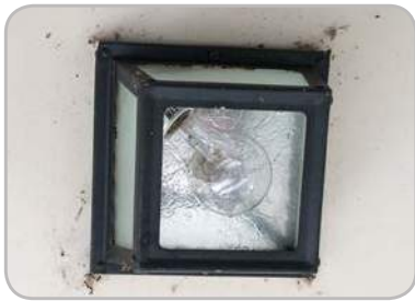
Figure 35: UNO should replace all incandescent bulbs, like this one at University Village, with CFLs or LEDs. The payback period for a CFL is typically less than 12 months while the payback period for a LED can range from 12 - 36 months.
