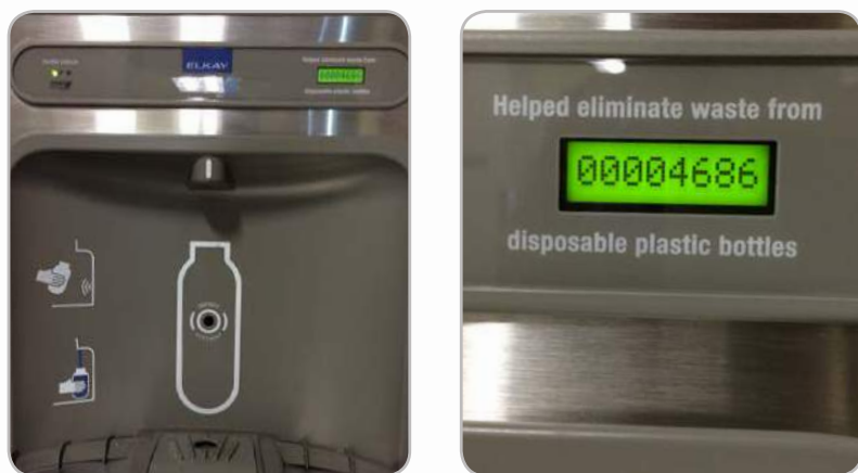
Figures 47 & 48: UNO has added several water bottle refill stations across campus. Students and employees enjoy using the stations because they help eliminate waste in the form of disposable plastic water bottles. In fact, each station displays a running count of how many disposable plastic water bottles it has displaced.
