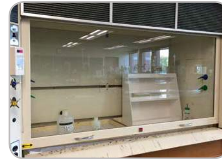
Figure 38: Another energy-saving opportunity is for campus users to appropriately shut fume hoods to minimize unnecessary ventilation
