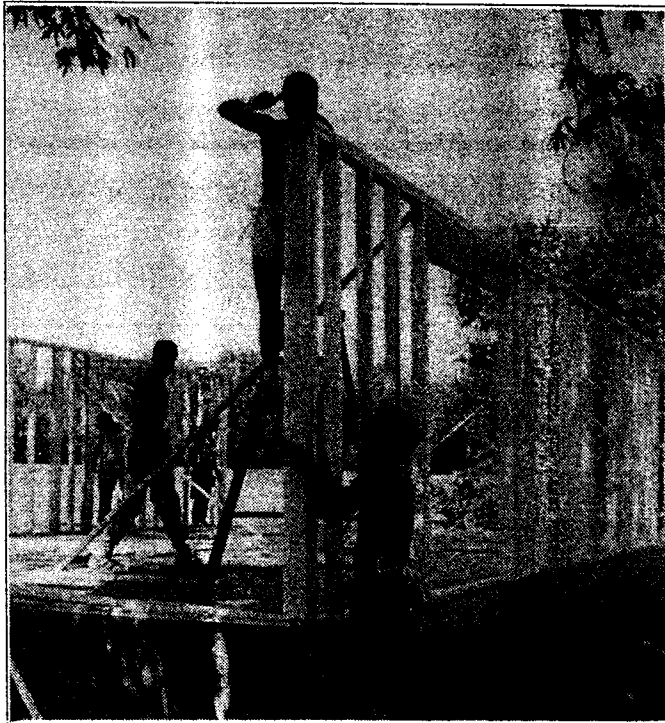
After a period of planning with Habitat for Humanity, young members of church groups in Evansville, Florida erected three homes in a four-day period. The houses will be given to low-income families.
