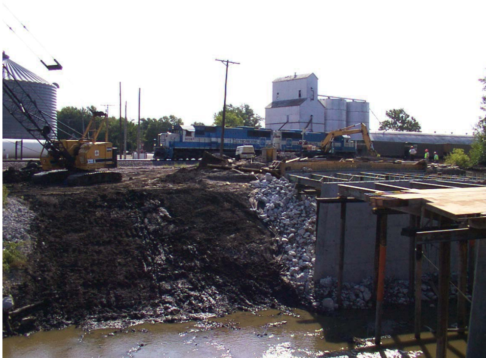
FIGURE 2 A railroad crossing is located immediately following the end of the bridge.
