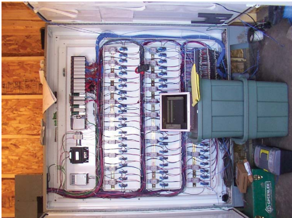
FIGURE 12 Microprocessor-based controller system.
