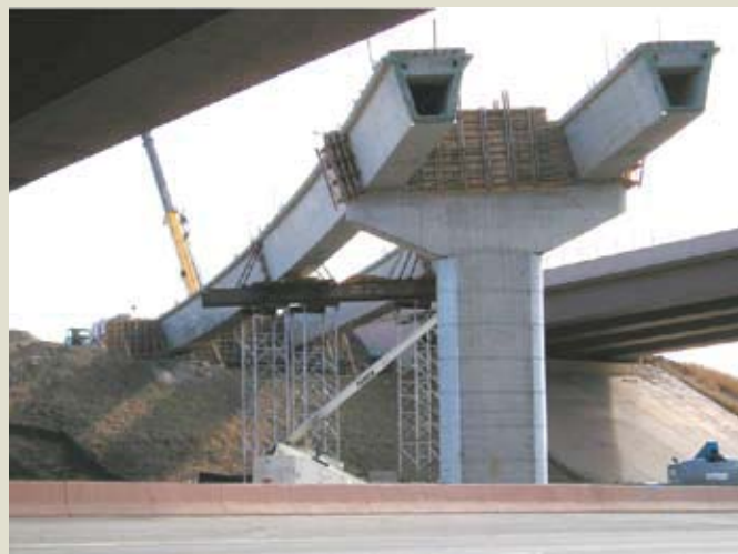
Figure 5. The 100-ft-long segments were cantilevered from the piers and supported by temporary shoring for the Interstate 270 bridge in Denver, Colo. Note: 1 ft = 0.305 m. Courtesy of Gregg Reese, Summit Engineering.
