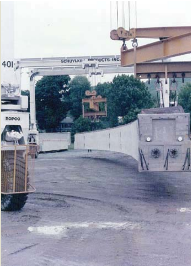
Figure 2. The Pennsylvania Department of Transportation used curved, precast, post-tensioned concrete box girders produced by Schuylkill Co. for the Philadelphia Airport renovation. Courtesy of Joseph Nagle, Schuylkill Co.
