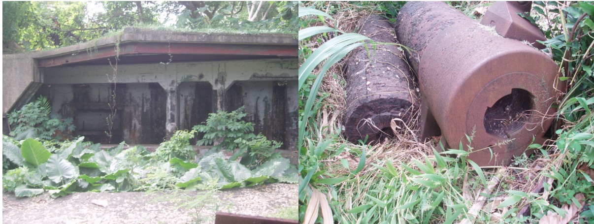
Images 6 and 7: The Flagstaff Battery, Pieces of the guns on the ground near the structure
