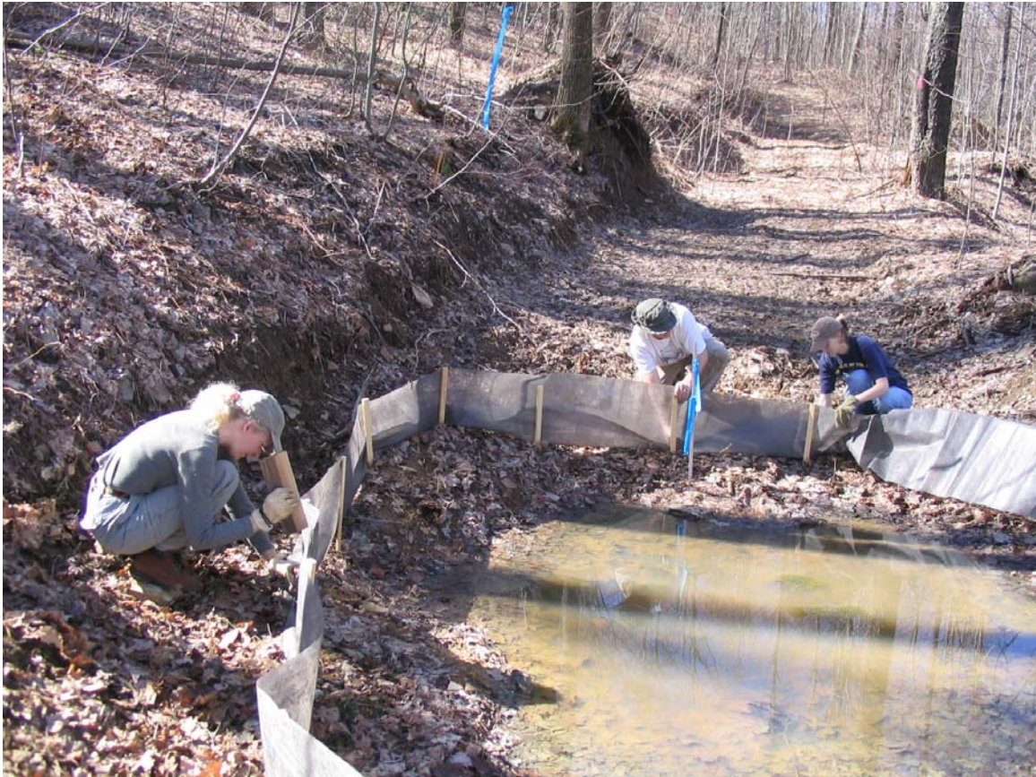
Figure 15. Installing silt fencing onto wooden stakes to completely encircle Pond 2 at Site 1 (March 2005). (Photo by: Becky Murray)
