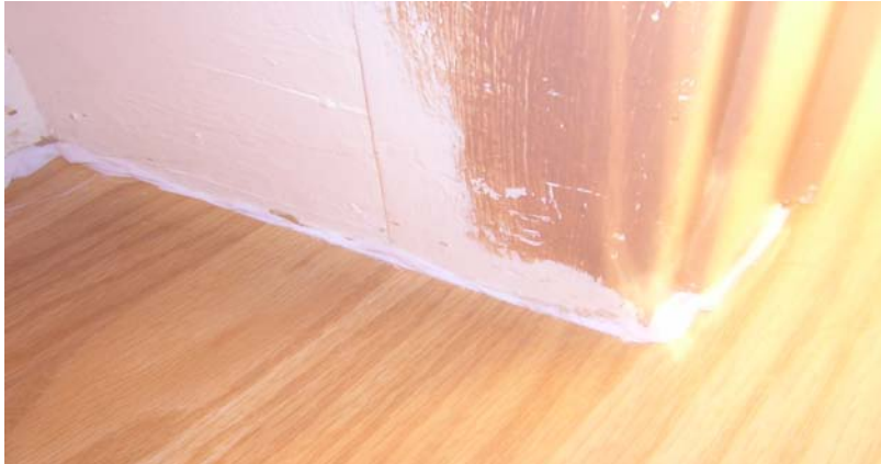
Figure 9. Crack filled with toilet tissue
