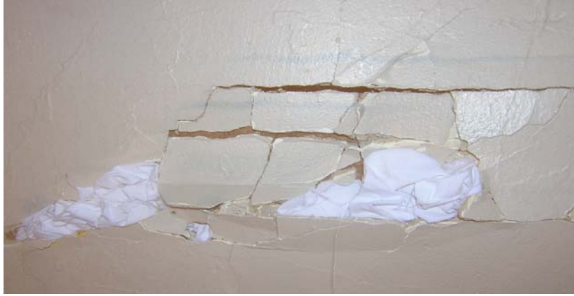
Figure 11. Hole in closet carefully stuffed with cloth
