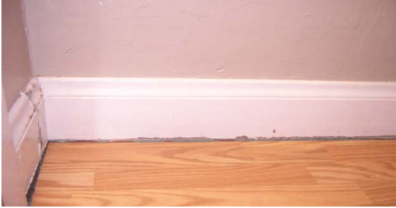
Figure 8. Crack between floor and wall
