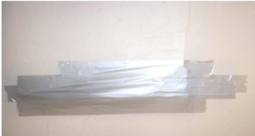
Figure 12. Hole in closet sealed with duct tape
