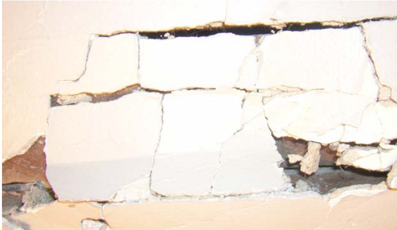
Figure 10. Hole in closet wall
