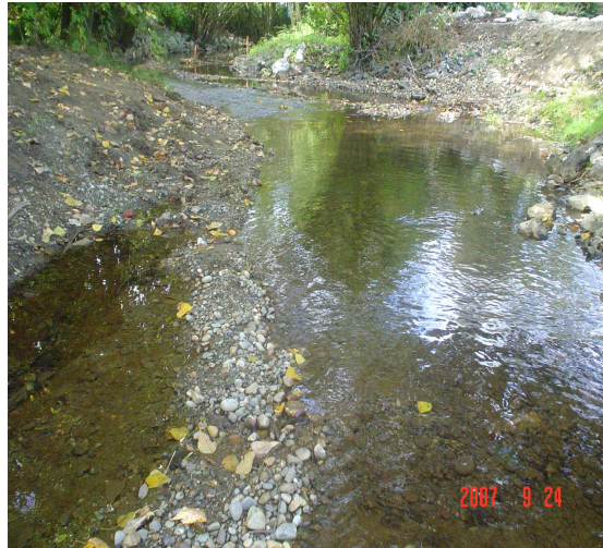
Figure 7. Same portion of channel as in Figure 6, illustrating the dredging done by the City of Abbotsford in fall 2007.
