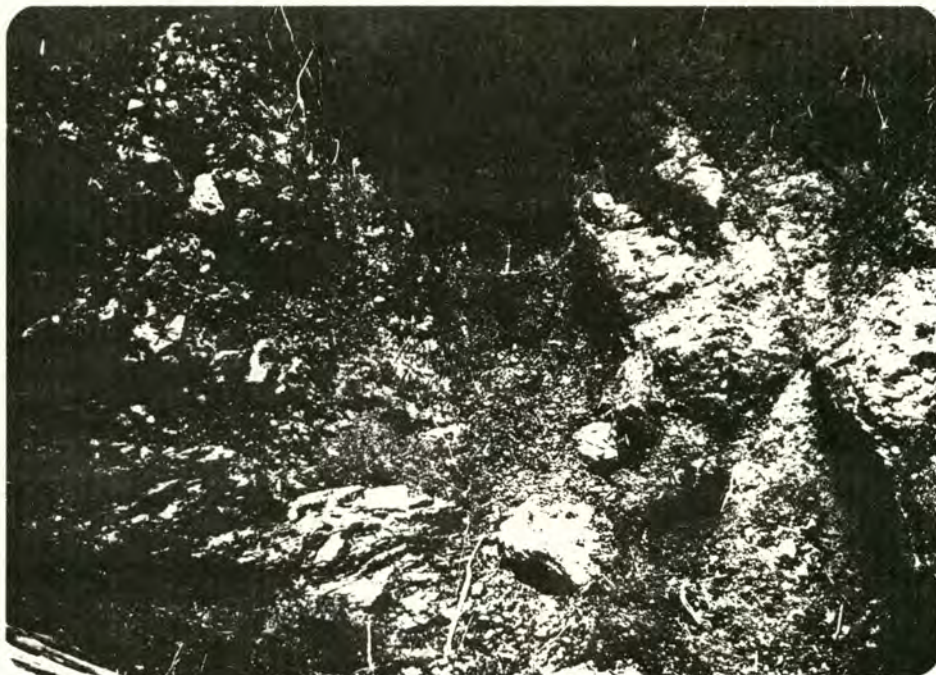
PLATE 17. Gouge zone in a fault between the rocks of Frailey Mountain on the left and Bulson Creek rocks on the right. Photo taken south of Lake Cavanaugh.
