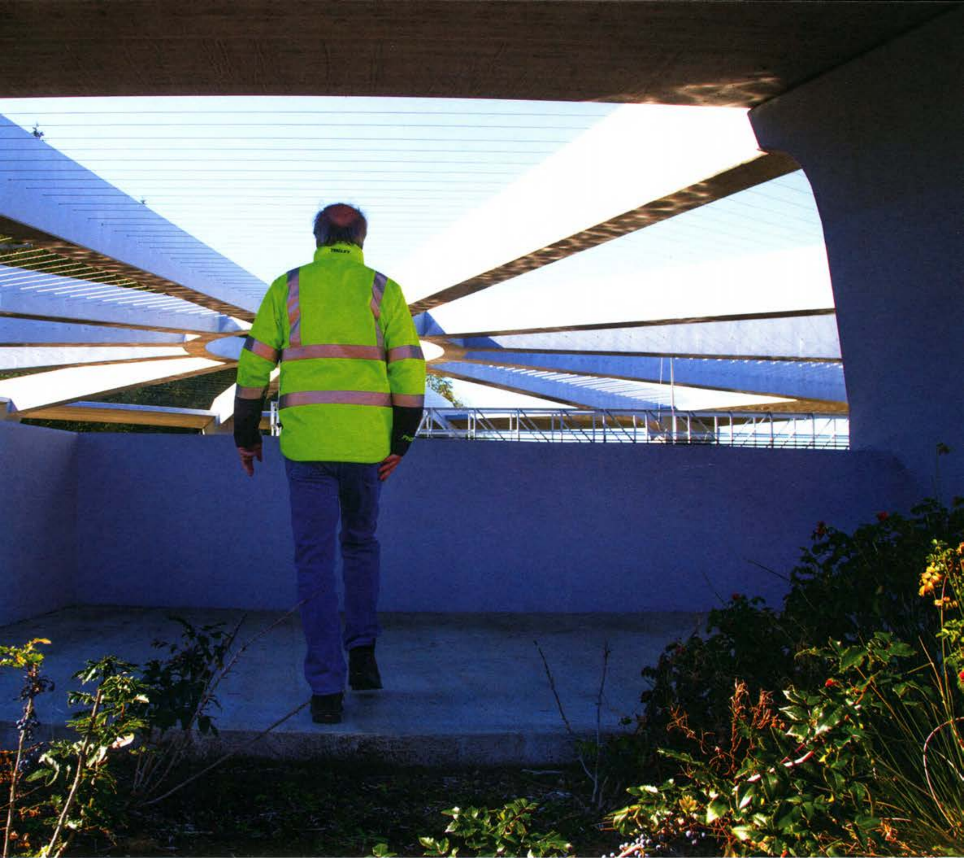
ABOVE: Operations supervisor Karl Lowry walks toward the clarifiers at the Post Point Wastewater Treatment Plant in Bellingham, Washington. The clarifiers sink solids in the wastewater to the bottom.
