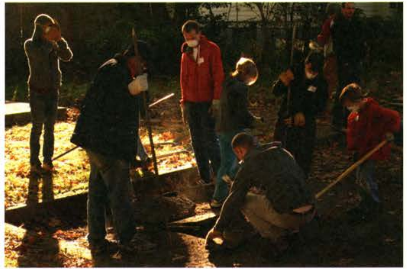
▲ About 25 volunteers showed up at the Southeast Uplift Center on October 16th to help remove unnecessary pavement from part of the center's parking lot.
