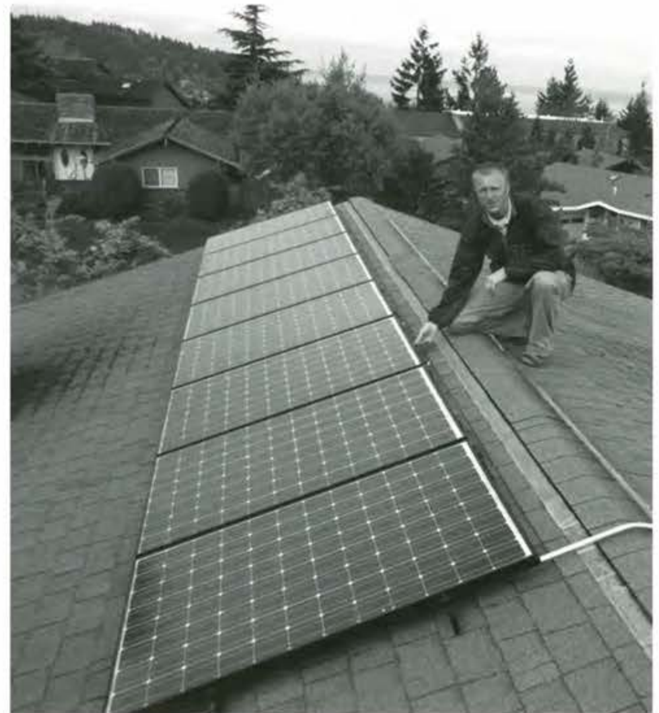
Dana Brandt, owner of EcoTech Energy systems, displays solar panels that have been installed on the roof of a local Bellingham residence.
