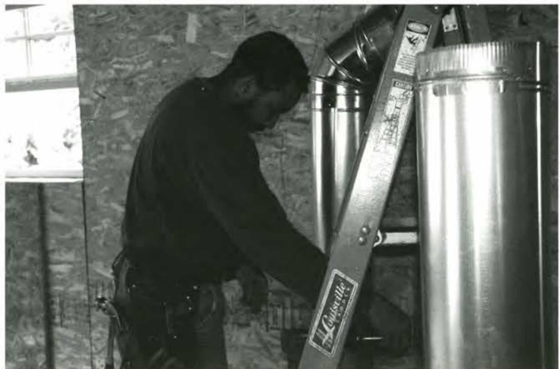
[Above] Andgar Heating installer, Chris Paris, works on installing a heating unit in Andy Walker's house.
