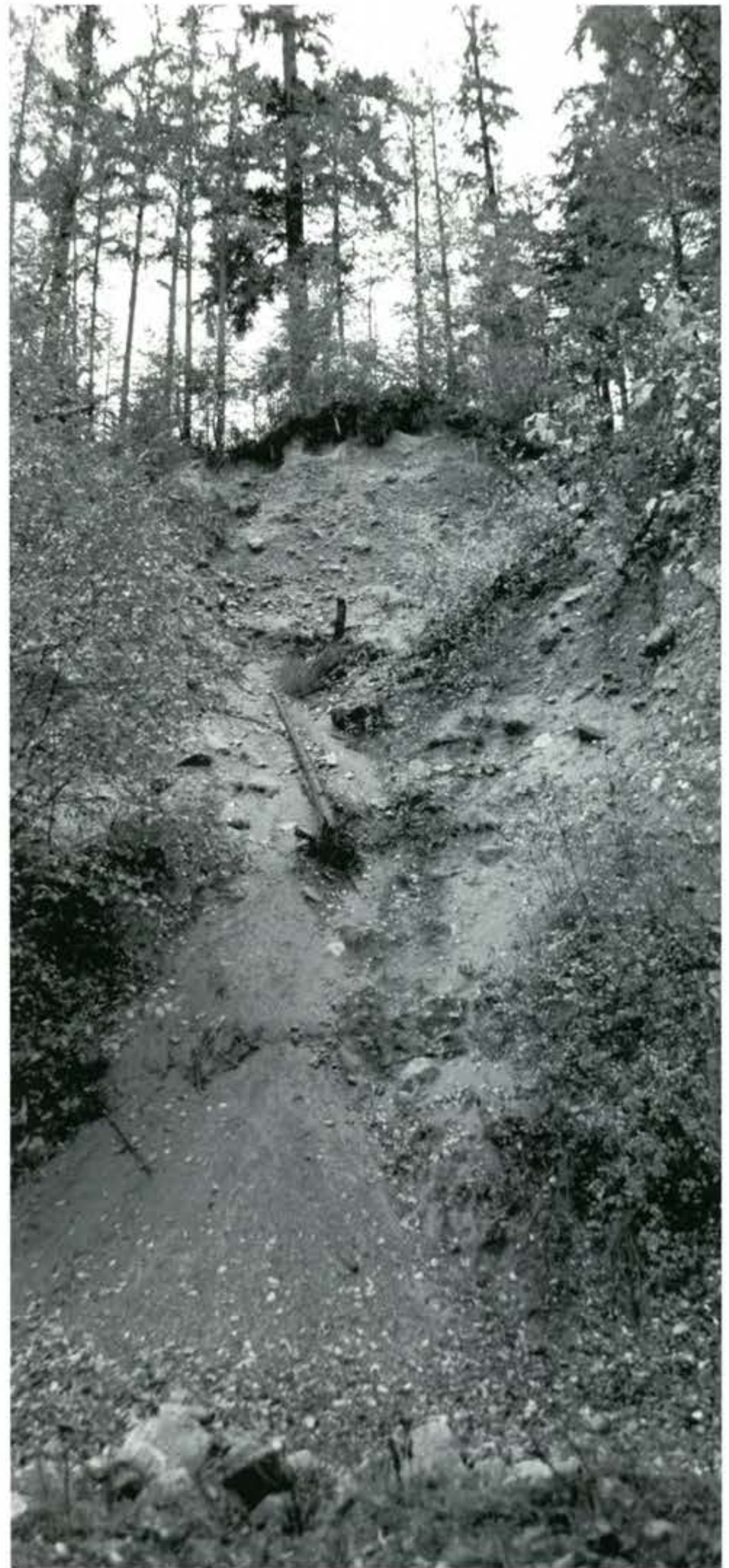
Mudslides continue to occur along Cascade River Road outside of Marblemount, the site of the 1985 fatal slide. Photo by Katie Kulla.
