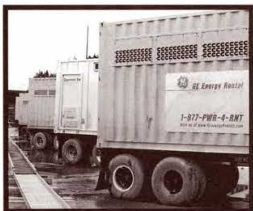
Photo by Nathaniel Fisher. Forty trailers hold diesel generators in the G-P parking lot.
