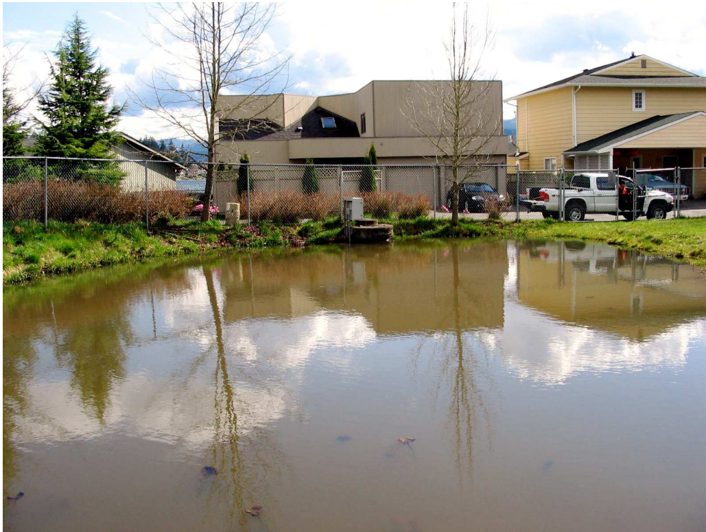
Figure A7: Photograph of the original Park Place storm water treatment system prior to retrofit (March 2005).
