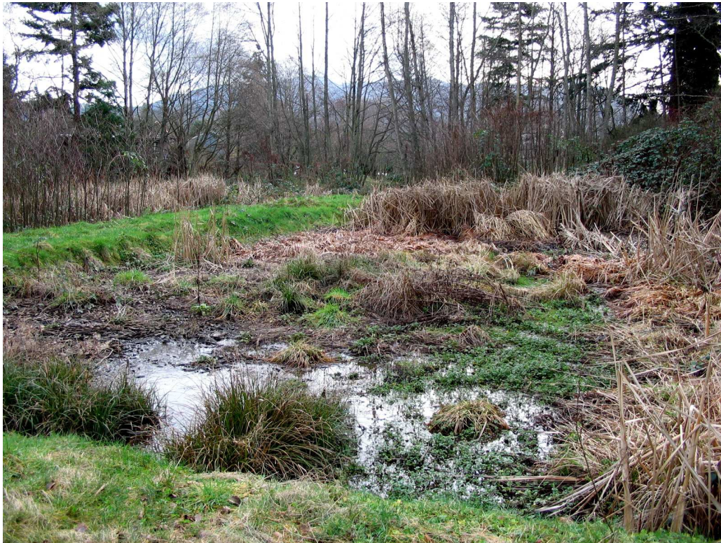
Figure A11: Photograph of the South Campus storm water treatment facility, January 2005. This site was not sampled in 2008/2009.
