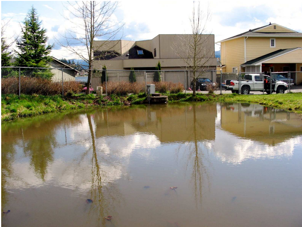
Figure A8: Photograph of the original Park Place storm water treatment system prior to retrofit (March 2005).
