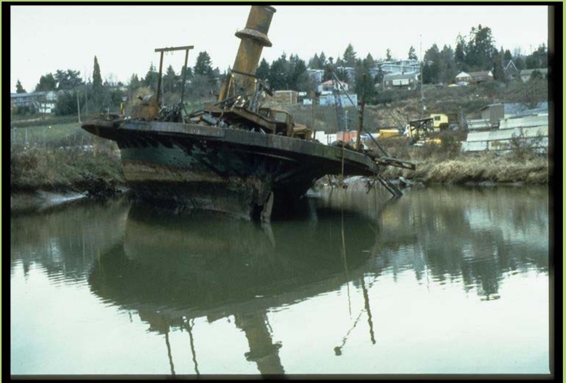
Removal of derelict vessel at Turning Basin Number Three, as portion of Terminal 5 redevelopment environmental restoration.
