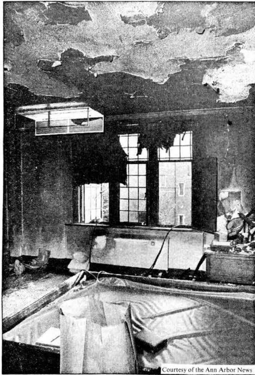
The charred remains of Picozzi's room after the blaze.
