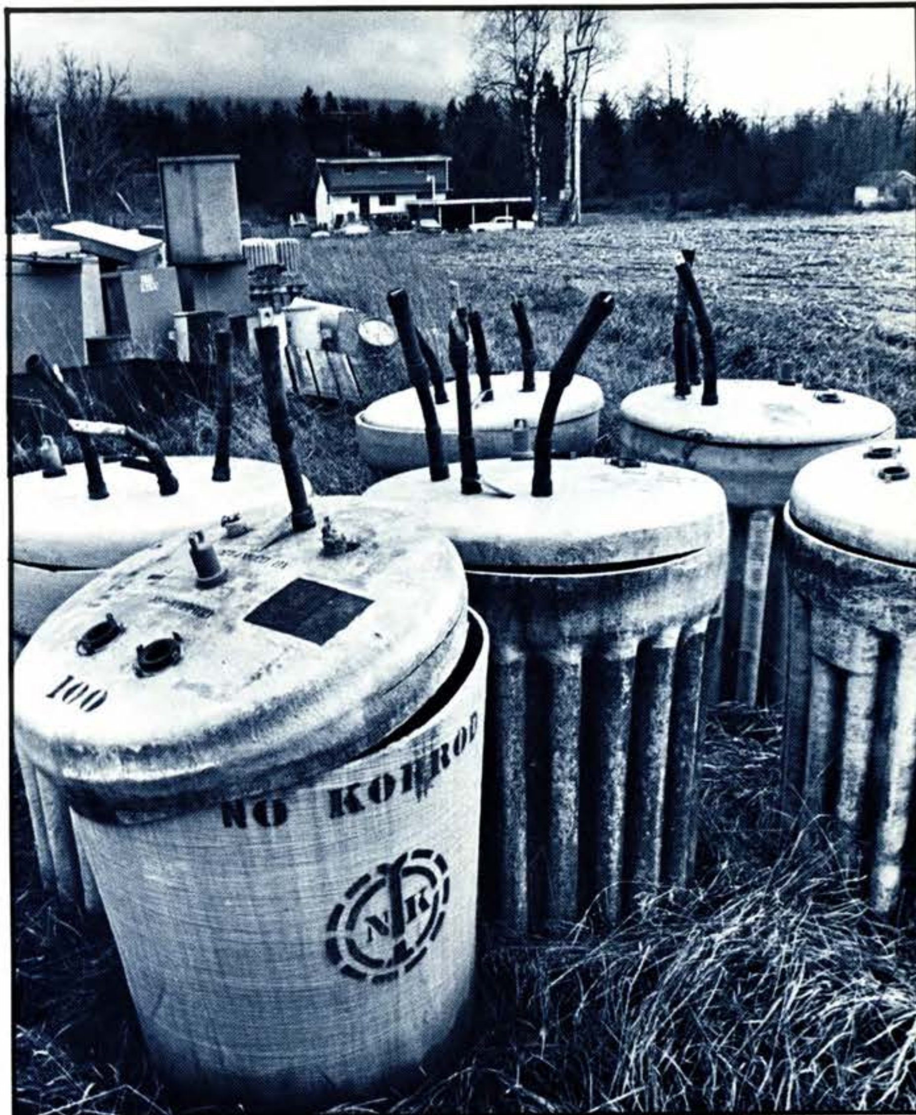
The transformer site is bounded by corn fields on two sides. Neighbors say the corn is used for fodder.
