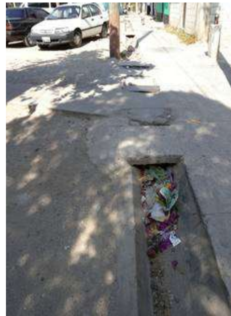
Figure 14. Trash accumulation in drainage ditches.
