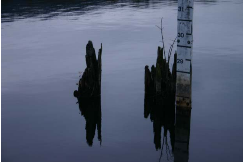
Photo 4 Deteriorated creosote pilings next to a water level marker.
