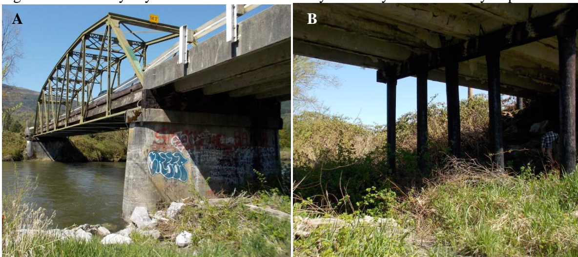
Figure 12: A. Concrete columns in the South Fork and B. creosote pilings on the east side of the river. Removal of these structures could increase sediment flux to the river if not dismantled carefully.
