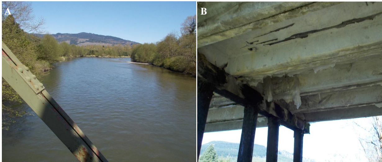
Figure 17: A. Scenic view of the South Fork Nooksack River, looking downstream from the Potter Road Bridge. Note the peeling paint on the cross-beam in the foreground. B. Underside of the bridge's eastern side, with creosote pilings and tattered plastic.
