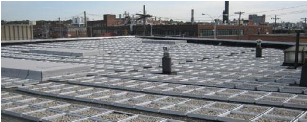
Figure 5: A modular blue roof installation [6]
