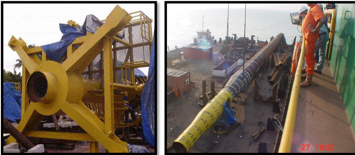
Figure 11 - (Left) Platform assembled onshore. (Right) Monopole being transported to site. [Photos courtesy of Dr. Anil Patnaik, The University of Akron]
