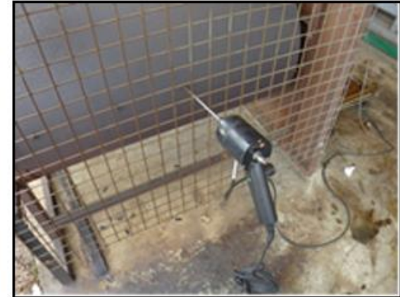
Gas sampling probe (flue gas)
