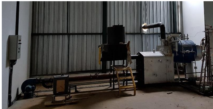
Biomass combustion laboratory
