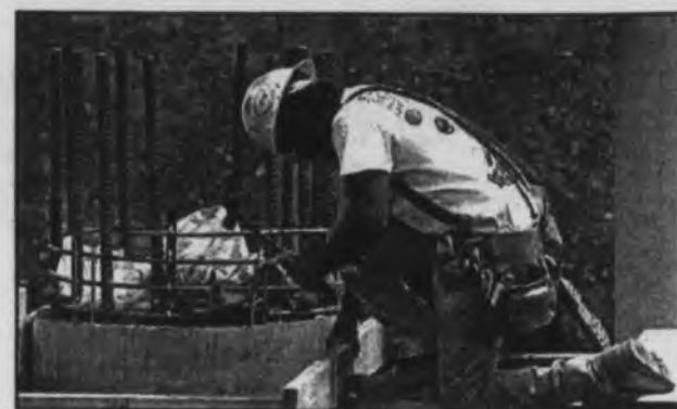
Lonnie Lewis of Richmond works on the new bridge being built over I-75 on Barnes Mill Road. A new bridge will be built and the old one will be torn down then rebuilt to make a four lane bridge across the interstate.
