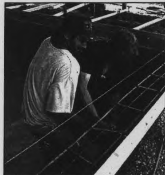
Anthony Wade (left) and Price Harrison are hard at work installing the pool in the new Hampton Inn.
