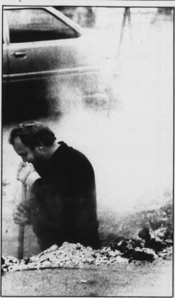
Feeling the heat Bobby Alexander, a university plant employee, works on a ruptured steamline pipe in front of the Moore Building.
