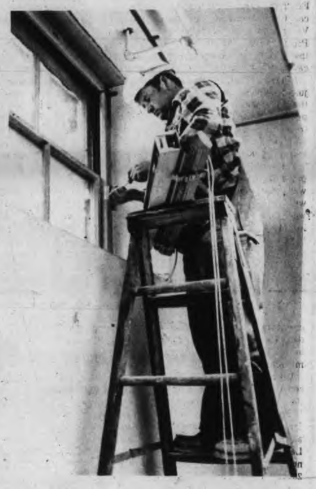
In order to remove any obstacles in the interior renovation of the Cammack building.
