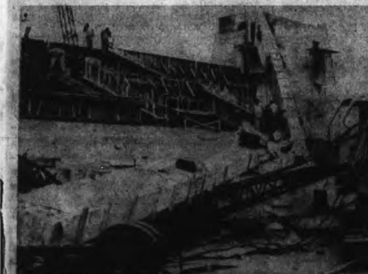
FALLEN ARCHES... The destruction dealt by the collapse of the two huge laminated arches at the Alumni Coliseum construction site this summer is shown close-up in the above photograph. Note the cab of the crane, in which a workman was seated during the fall, was in the direct path of the falling arch. The mangled boom of the 25-ton rig was estimated to be a loss of about $25 thousand. Behind the crane a quarter section of bleachers was demolished.
