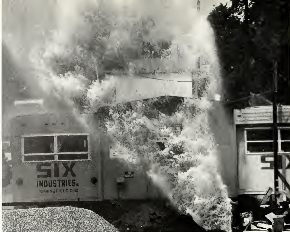
A ruptured water main delays construction on the Jane F. Campbell Building. Right: Construction workers stand idle awaiting repair of the broken water main.
