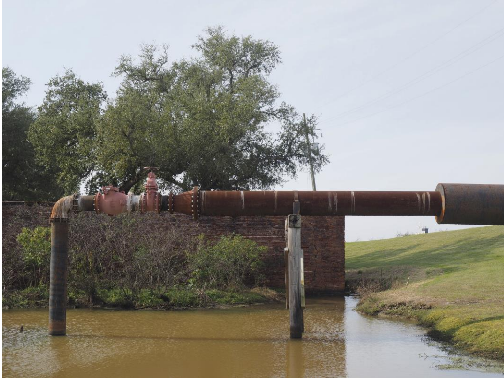
15. Flood / rainwater drainage at Fort Jackson, Plaquemines Parish.
