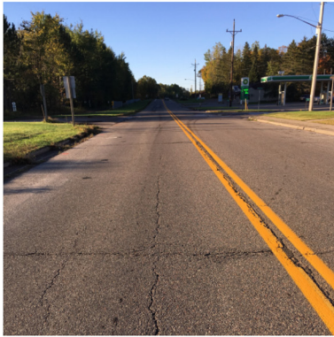
a) Pavement surface distresses
