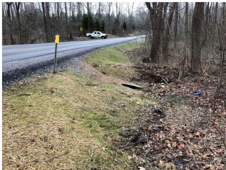
Figure 9 Depression Above Pipe
