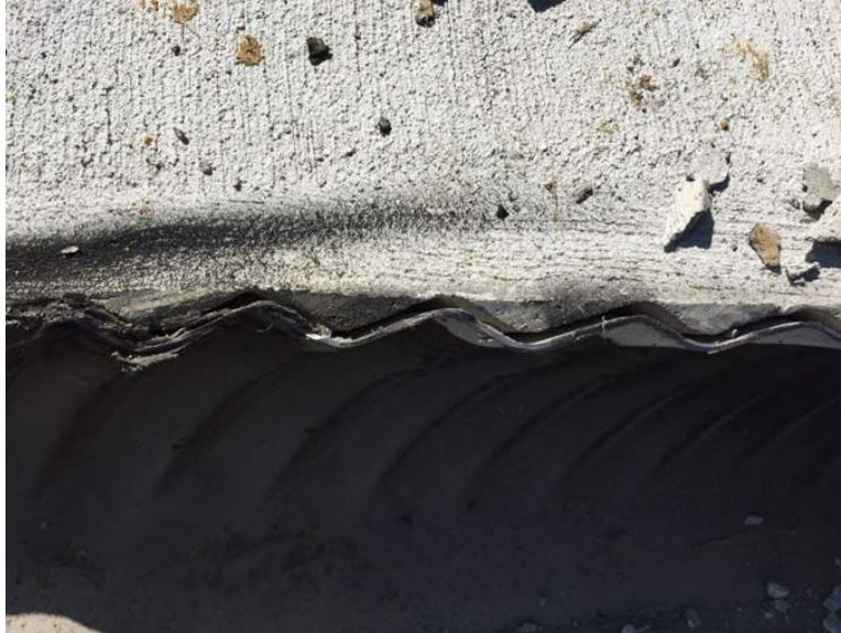
Figure 4 Separation Between Headwall and Pipe End
