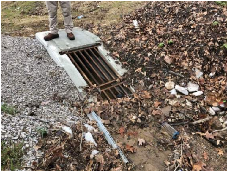
Figure 10 Safety Type Box Inlet Grate Blocked
