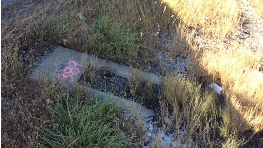
Figure 3 Outlet Waterway Blocked by Gravel
