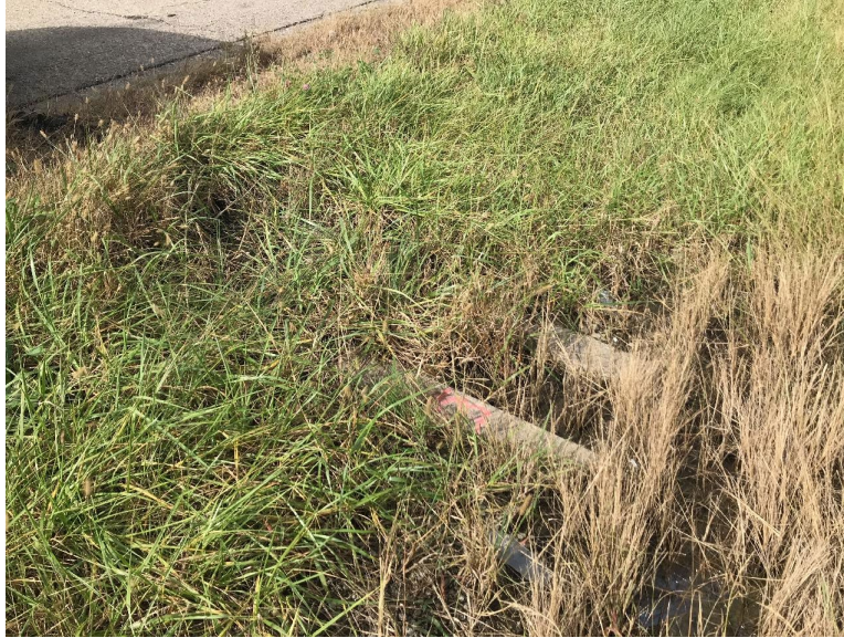
Figure 1 Outfall Waterway Obstructed by Vegetative Growth
