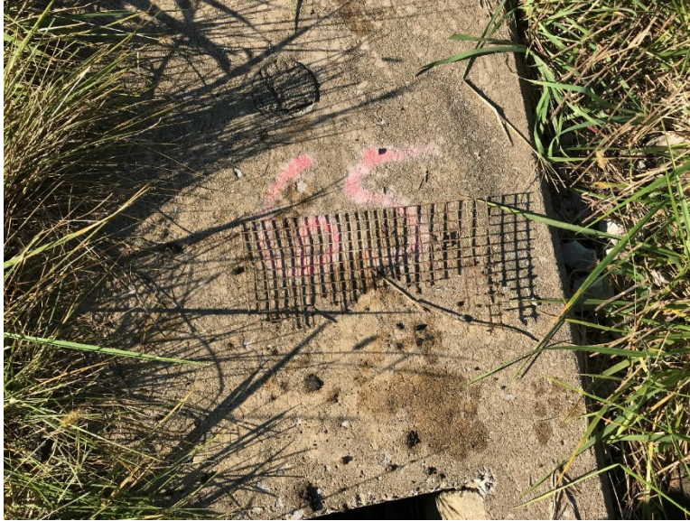
Figure 9 Rodent Screen Rusted Through
