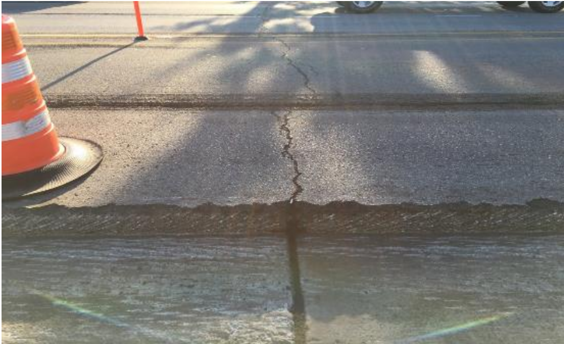
Figure 1 Example of Reflective Cracking
