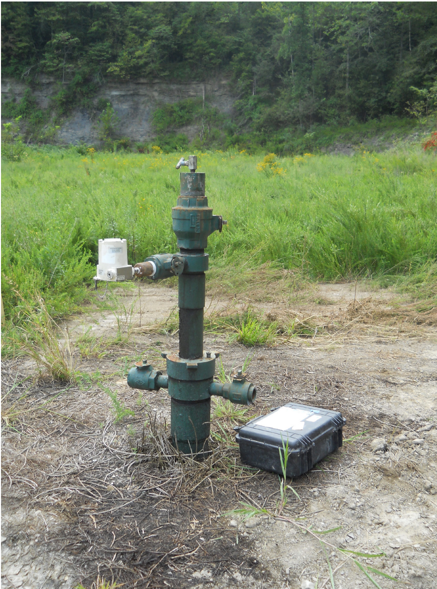
Figure 20. Typical installation of a surface data logger on the wellhead of the SS-#4 well.
