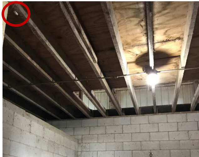
Figure 2.8 Openings in the ceiling of the stalls and location of the temperature and relative humidity sensor in the front left corner of the ceiling of the stall (Circled in red).
