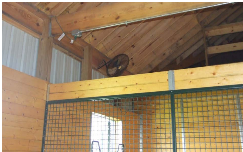
Figure 2.2 Overhead fan in the eaves blowing down into the stall.
