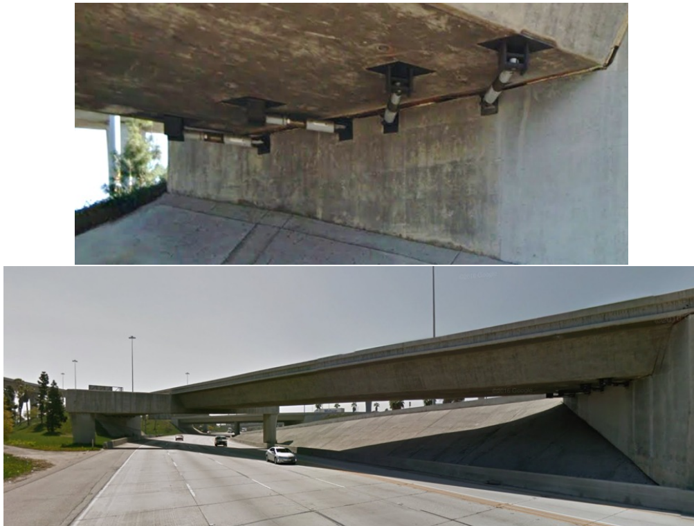
Figure 5. (a) Hydraulic dampers installed in the bridge case study. (b) Google street view of the actual highway bridge
