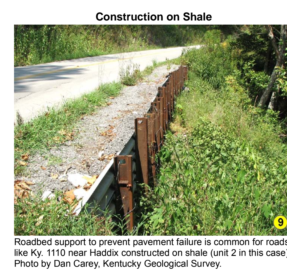
Construction on Shale Roadbed support to prevent pavement failure is common for roads like Ky. 1110 near Hadix constructed on shale (unit 2 in this case). Photo by Dan Carey, Kentucky Geological Survey.
