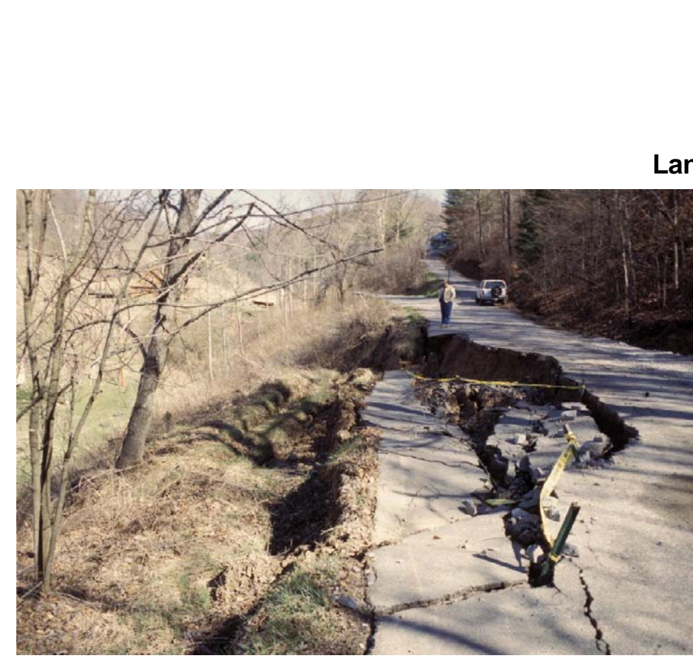
Landslides Hillslope construction can cause earth movements if not properly planned. Photos by Paul Howell, U.S. Department of Agriculture, Natural Resources Conservation Service.
