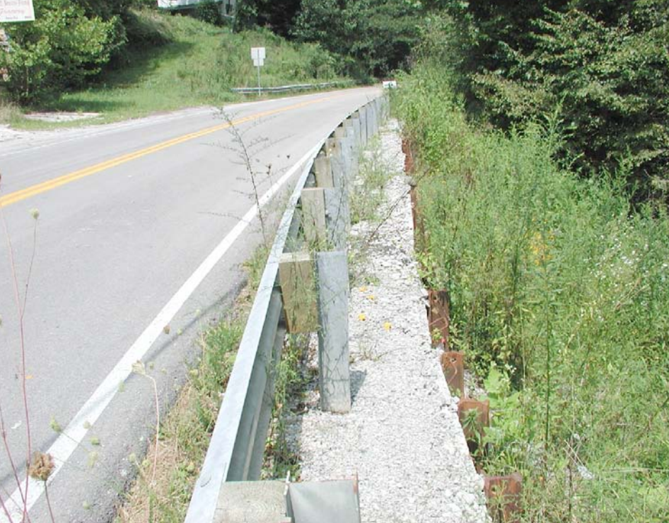
Drainage management and roadway support are mandatory in steep slope areas that are common in McCreary County, particularly if shale units are encountered. Photo by Randy Paylor, Kentucky Geological Survey.
