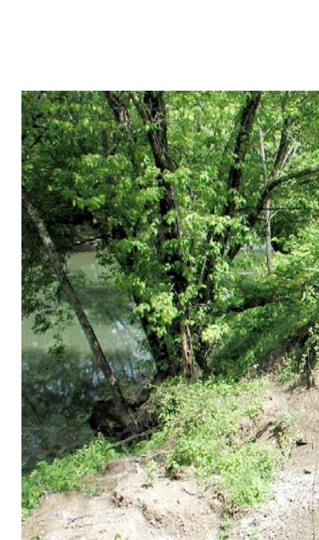
Road construction near stream banks and on hillsides can contribute to slope failure if not properly planned. Photos by Dan Carey, Kentucky Geological Survey.
