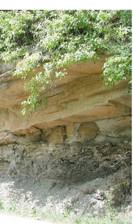
Construction at the interface of sandstone overlying shale presents possible rockfall problems as the shale erodes beneath. Photo by Dan Carey, Kentucky Geological Survey.
