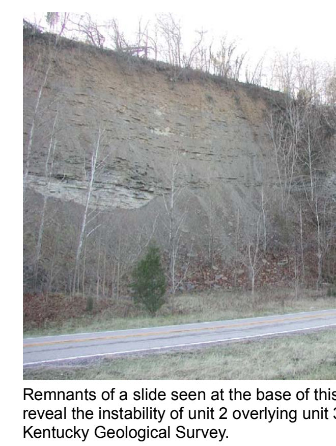
Remnants of a slide seen at the base of this roadcut along Ky. 9 remain the instability of unit 2 overlying unit 3. Photo by Dan Carey, Kentucky Geological Survey.
