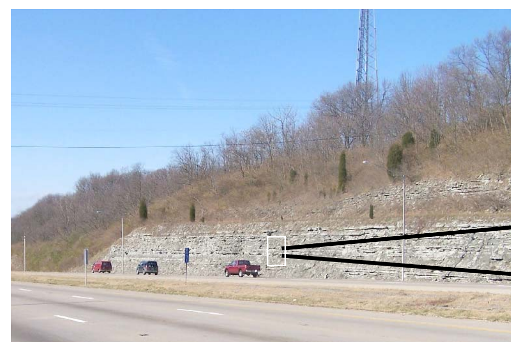
Limestone and shale (unit 3), the 500-million-year-old (Ordovician-age) Fairview Formation, is common as bedrock in Kenton County, and can cause problems for builders because the shales in the unit can swell when exposed to water. Photo by Richard Smath, Kentucky Geological Survey.
