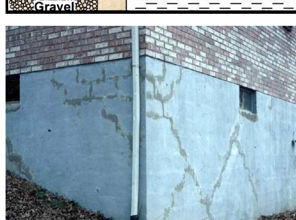
Some shales, and the soils derived from them, swell when exposed to water or air. These swelling shales and soils can have severe impacts on building foundations and other structures (e.g., bridges, dams, roads). Photo by John Kiefer, Kentucky Geological Survey.
