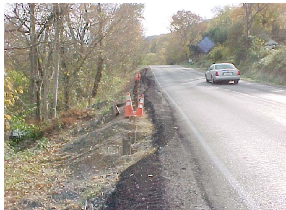
Slope failure along U.S. 42-127 east of Warsaw. The road is built on unit 2, and requires continued maintenance. The Ohio River is below to the left. Photo by Warren Anderson, Kentucky Geological Survey.
