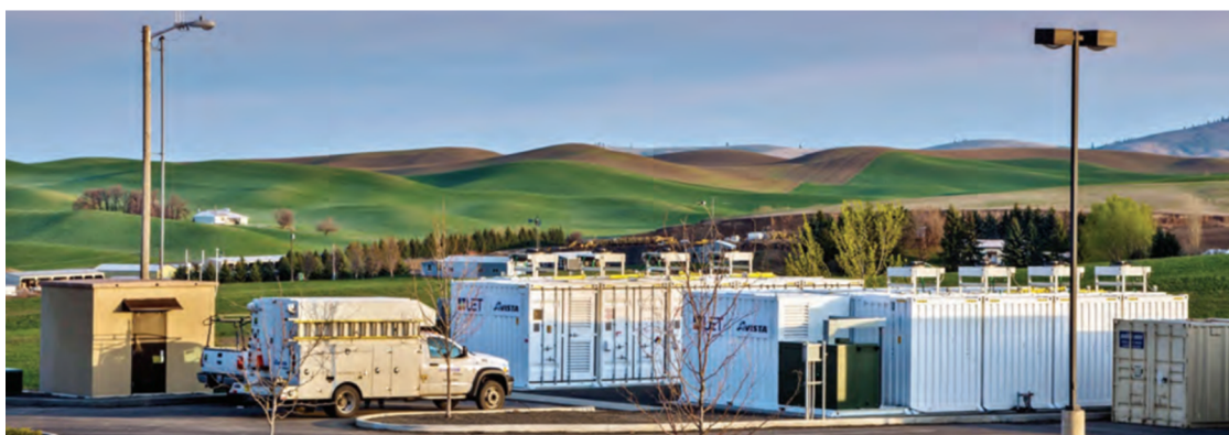
Figure 1. The 1 MW/4MWh Uni System installed at Schweitzer Engineering Laboratories in Pullman, Washington. Credit: http://uettechnologies.com .
