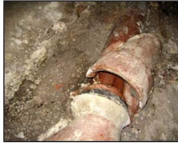
Separated sewer pipe
