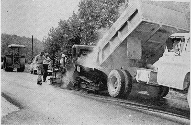
Fig. 5.—Paving operation on U.S. 60 in Rowan County. Conventional paving equipment and standard aggregate mixtures were used throughout the test projects.
