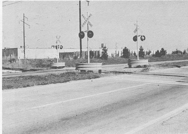
Figure 19. Improper use of guardrail.
