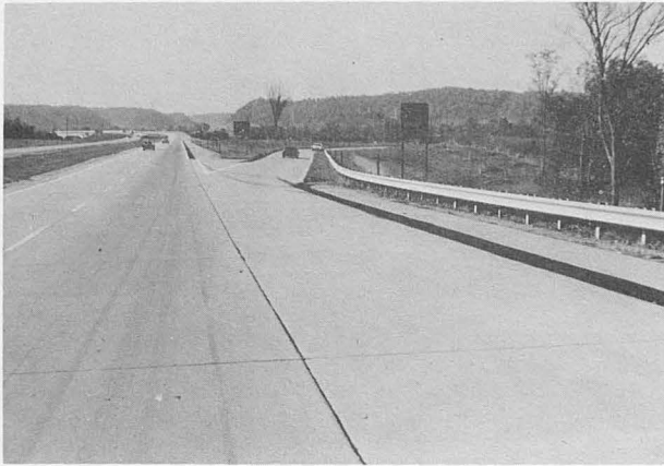
Figure 11. Discontinuous and improperly transitioned shoulder at exit ramp.
